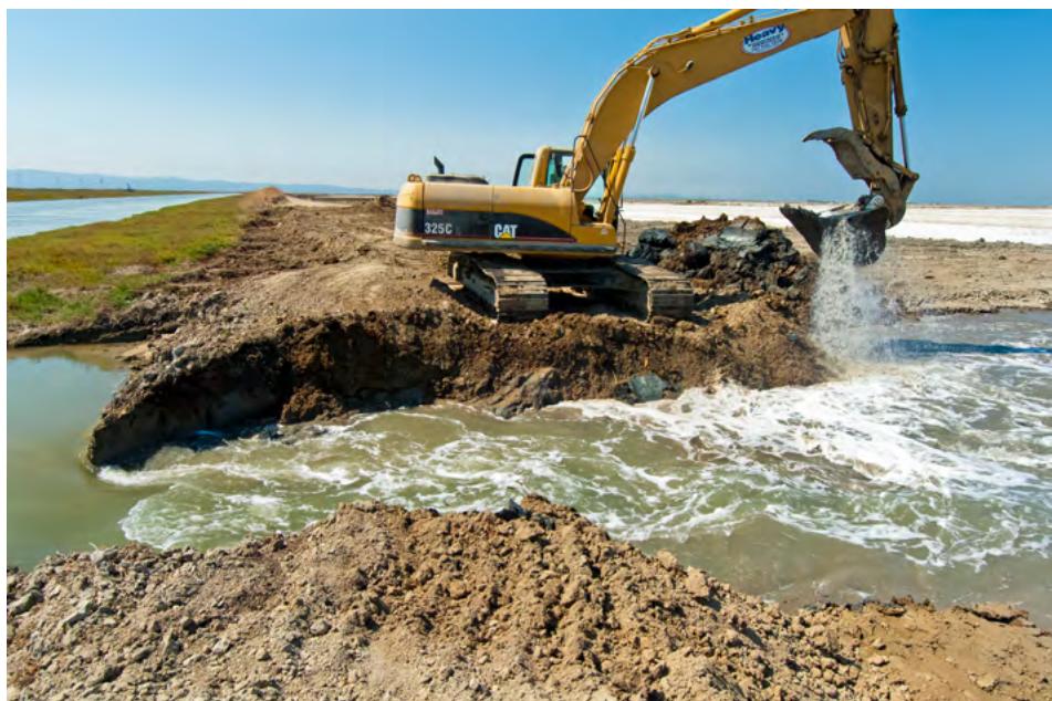
A 2010 levee breach reintroduced Bay waters to a former salt pond on the Don Edwards SF Bay National Wildlife Refuge. Photo: Judy Irving
